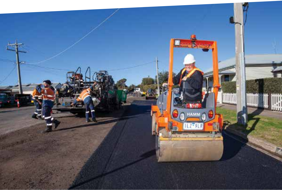
Mayor Cr Bob Merriman puts the finishing touches on the Bridge St resurfacing.
