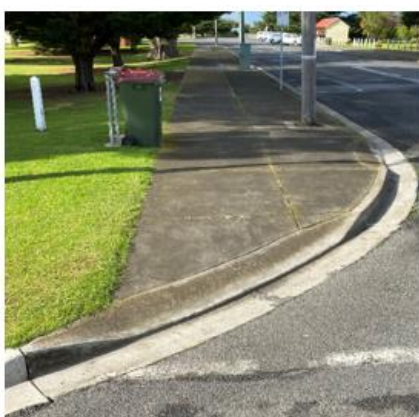
Non-compliant kerb ramp
