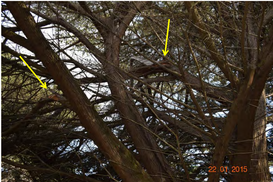
Figure 42: Many of the trees in this row have cracked or hanging branches above the shared path.
