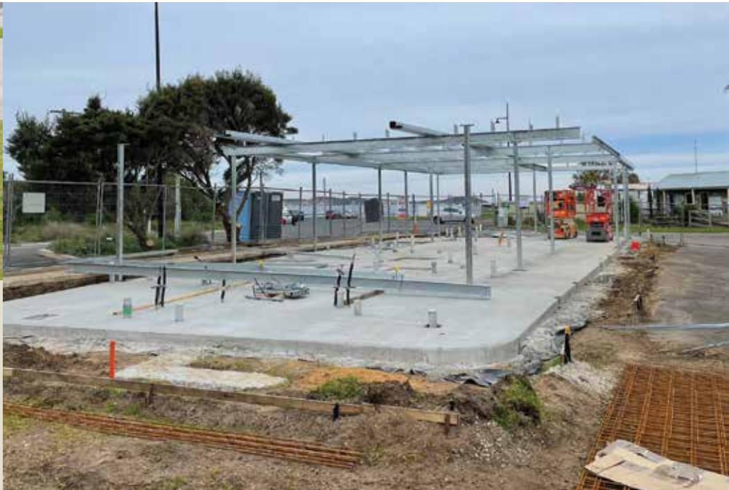
The construction site – with views of the water! – at the Queenscliff Recreation Reserve in late June.
