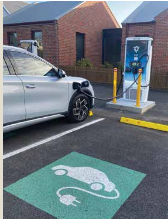
EV charging stations at Council Offices in Learmonth St. are now ready to charge.
